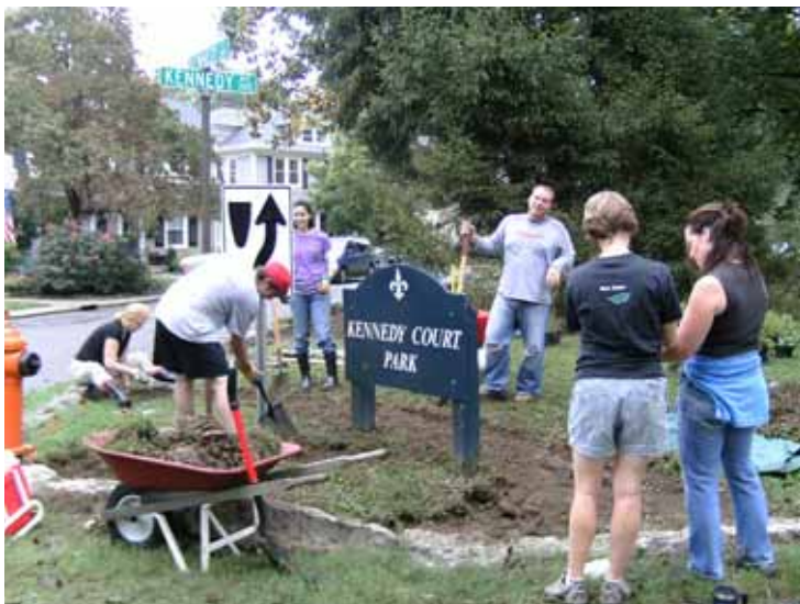
Homeowners in Kennedy Court work to install one of two rain gardens in their central park.
